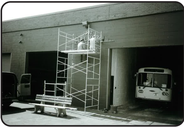
Sign being restored after blown down by wind (placed on lower building).
