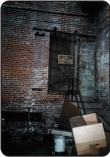
Inside of conference room in 2008 showing old fire door and junk.
